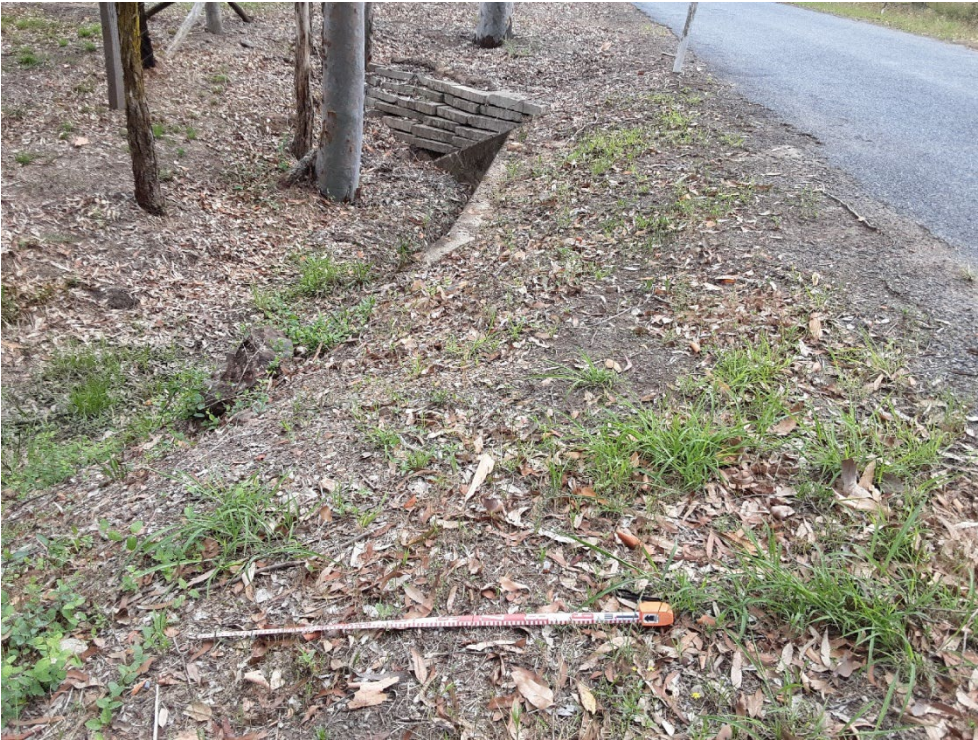
Photo 13 Northern portion of East Seaham Road, portraying a culvert located in the road corridor displaying 10% GSV
