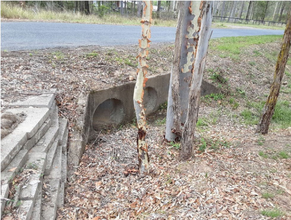
Photo 16 Example of drainage structures located throughout the study area, photo taken facing south-east
